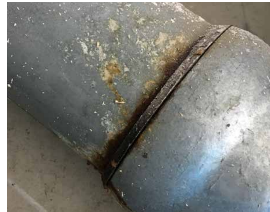
Corroded pipe connection in the steel pipe after around 50 years of use
