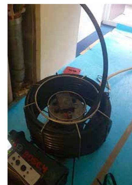
Using the cutting robot (IMS Robotics) in the DN 125 downpipe to open the inlets
