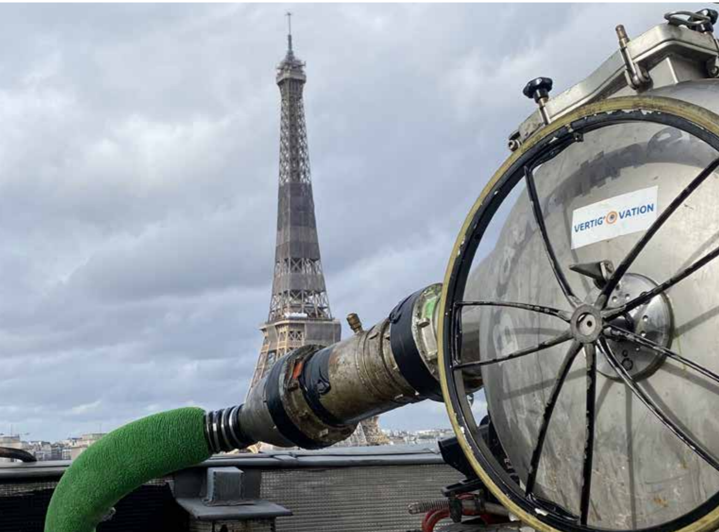
Magnificent view of the Eiffel Tower during the installation of the BRAWOLINER® HT DN 100
