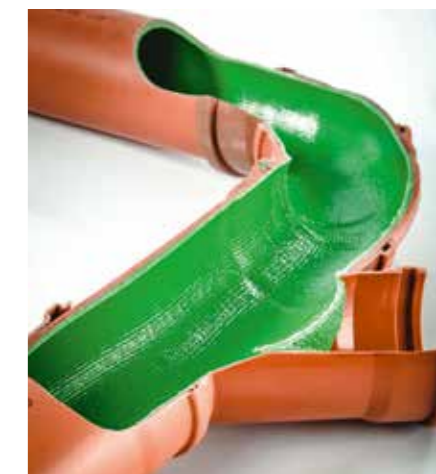
The pipes were mainly rehabilitated with the BRAWOLINER® HT. | Photo: Pipe Bull
