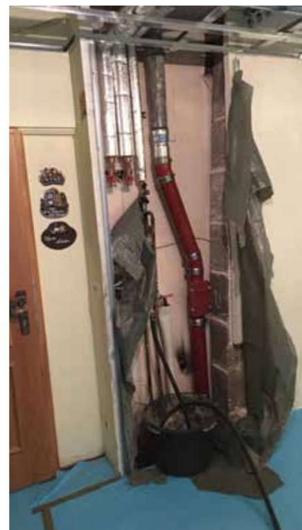
Newly created inspection openings on some intermediate floor levels of the holiday complex
